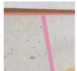
View of a properly sealed horizontal and vertical expansion joint in the wall
